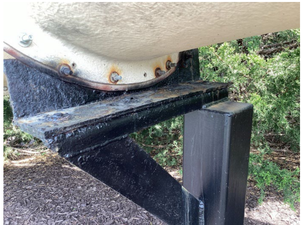
Rusted fasteners and bracket
