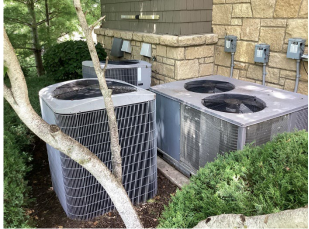
Split system condensing units
