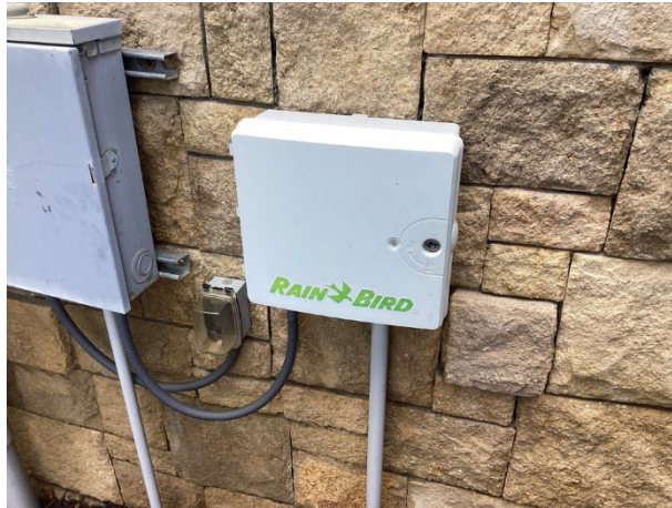
Irrigation system controller
