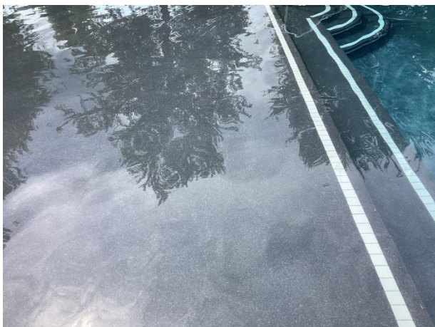
Plaster cracks at infinity pool
