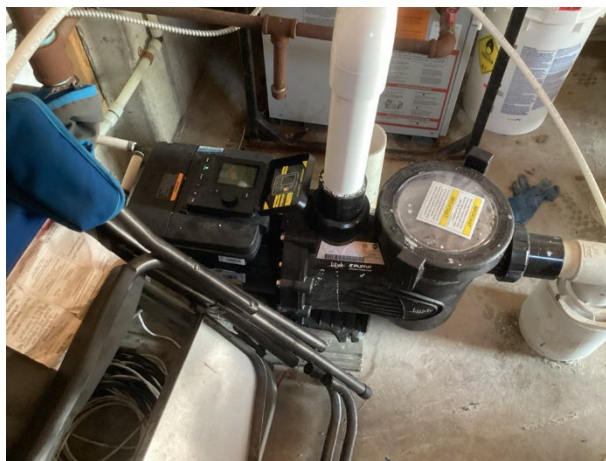
Water slide pump
