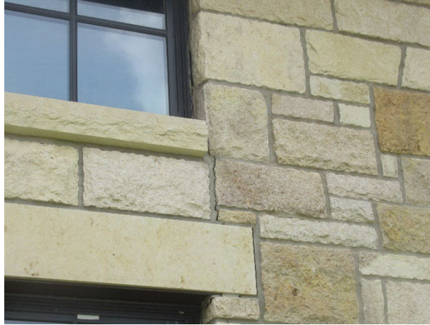
Mortar cracks at clubhouse
