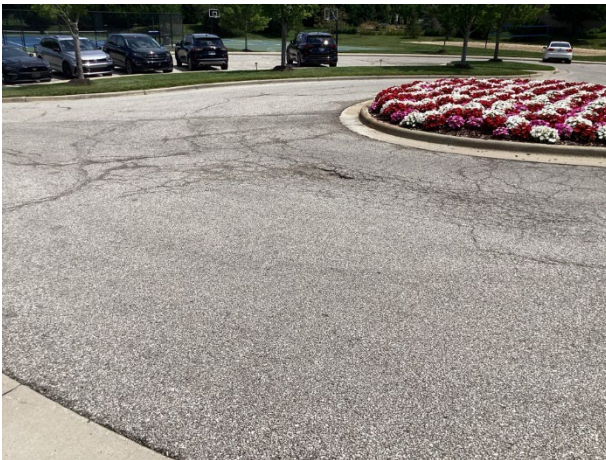
Pavement overview, note cracks and pothole formation
