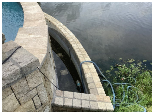
Current leak at infinity pool
