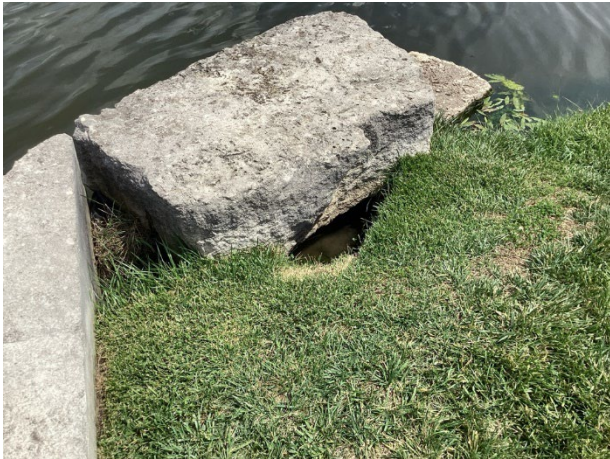
Erosion behind bulkhead by spillway
