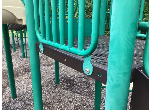
Equipment finish deterioration
