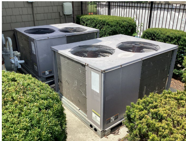
Split system condensing units
