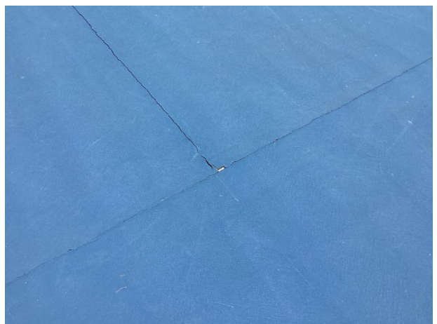
Surface coating cracks
