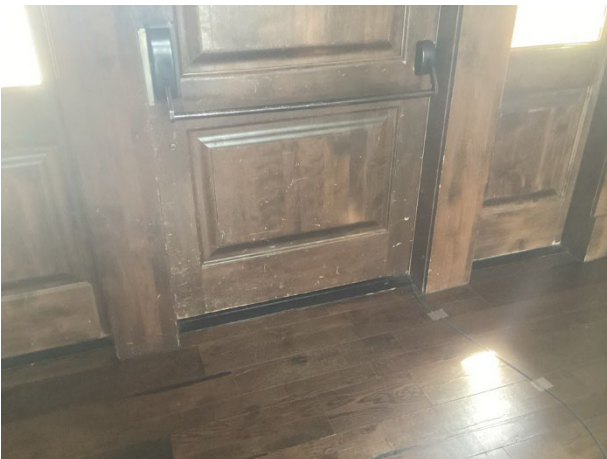
Main entry door finish deterioration
