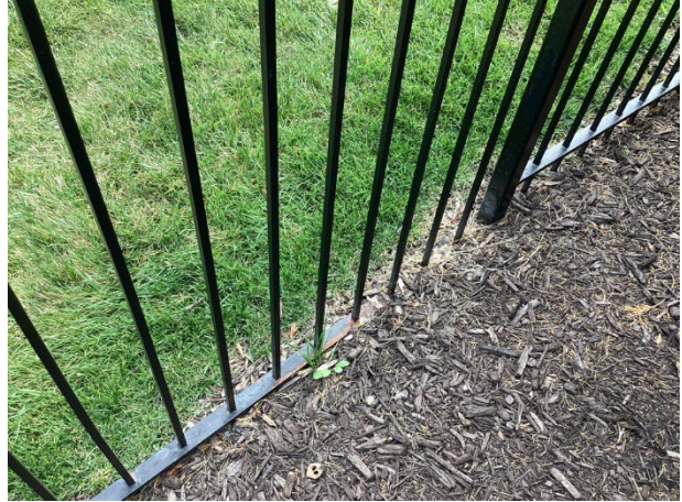
Fence finish deterioration
