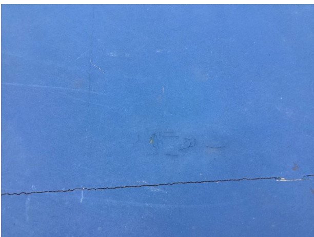
Color coat deterioration
