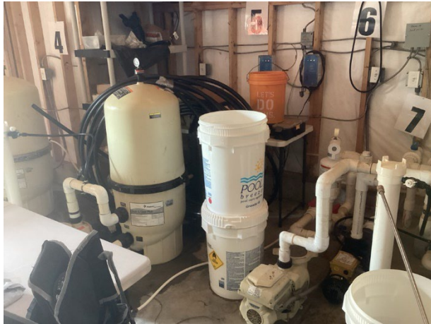
Pool mechanical equipment
