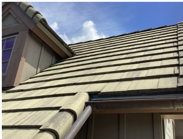
Minor damage at tiles
