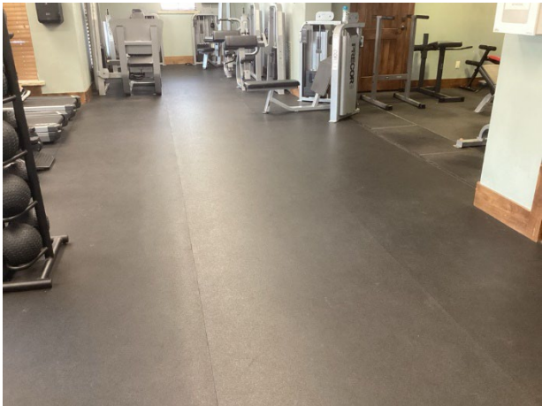
Exercise room flooring
