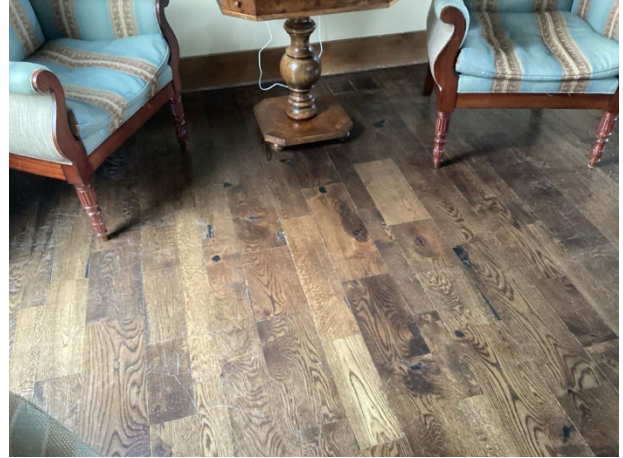
Worn furniture and scratches at wood flooring
