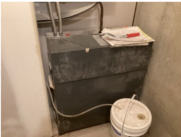
Hydraulic elevator equipment
