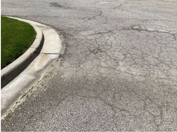
Alligator cracks and edge deterioration
