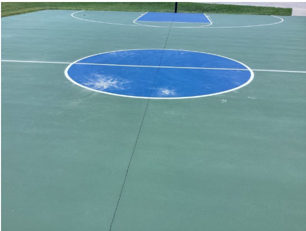
Basketball court overview, note surface crack along centerline joint
