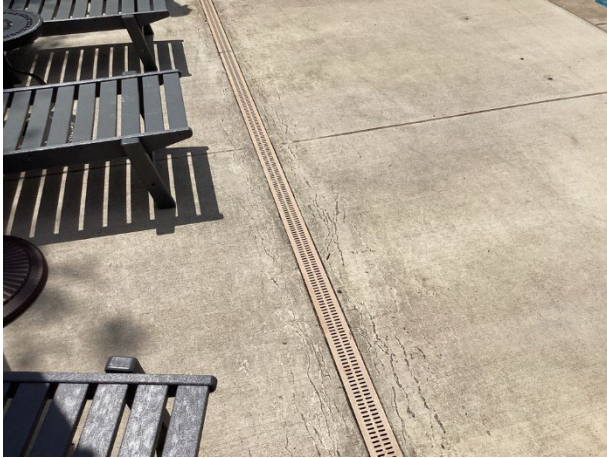
Concrete cracks along drain
